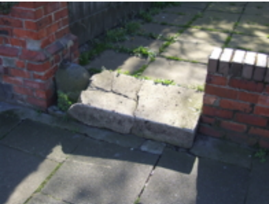
Broken step to northern boundary
