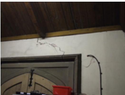
Cracking above and around East Aisle Store external doors
