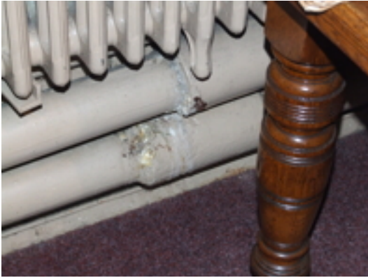
Leaking Heating Pipework
