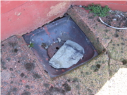
Sump with debris
