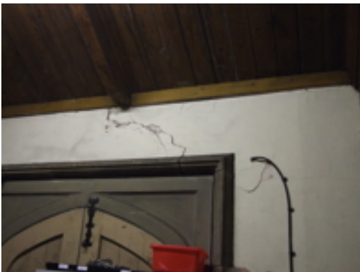
East Aisle Store cracking
