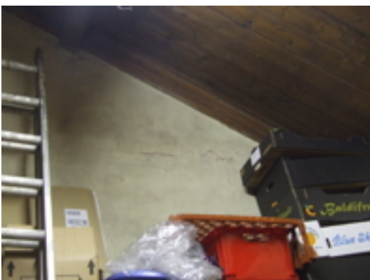
East Aisle Store loose plaster
