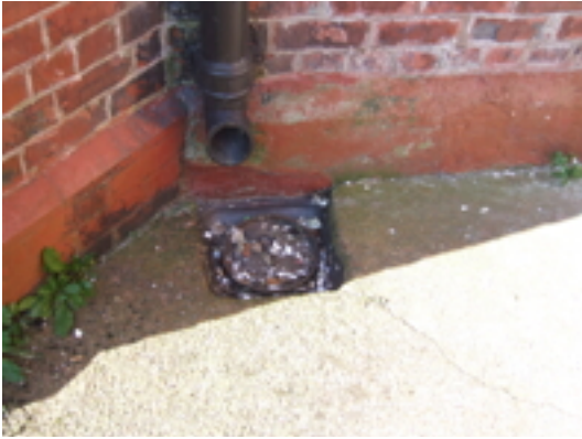
Sump with debris south east corner
