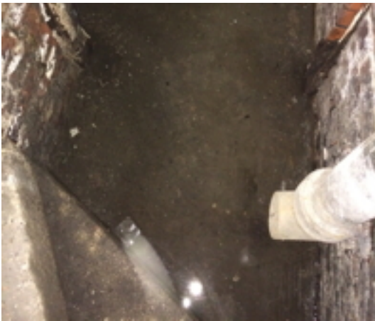
Boiler Chamber with blocked sump below redundant rainwater pipe.
