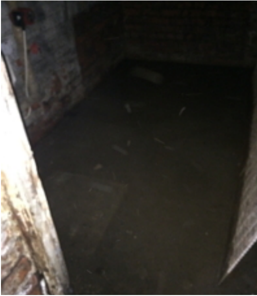
Boiler Chamber From Bottom of Staircase showing pump on west wall
