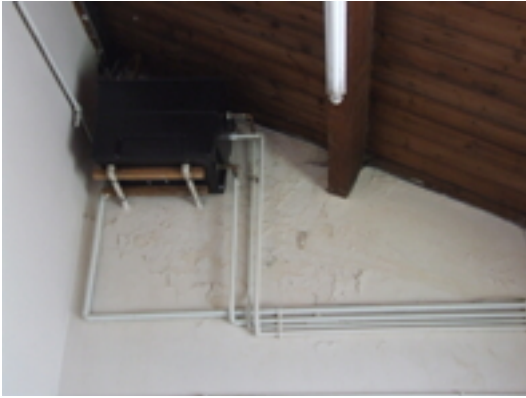
Flaking paint to Vestry north wall
